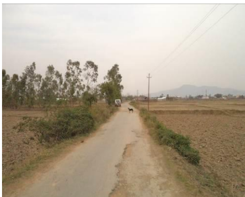
Road Condition of Sangaipour Village Road
